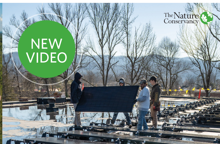
Middlesboro Community Center solar installation © Mike Wilkinson
