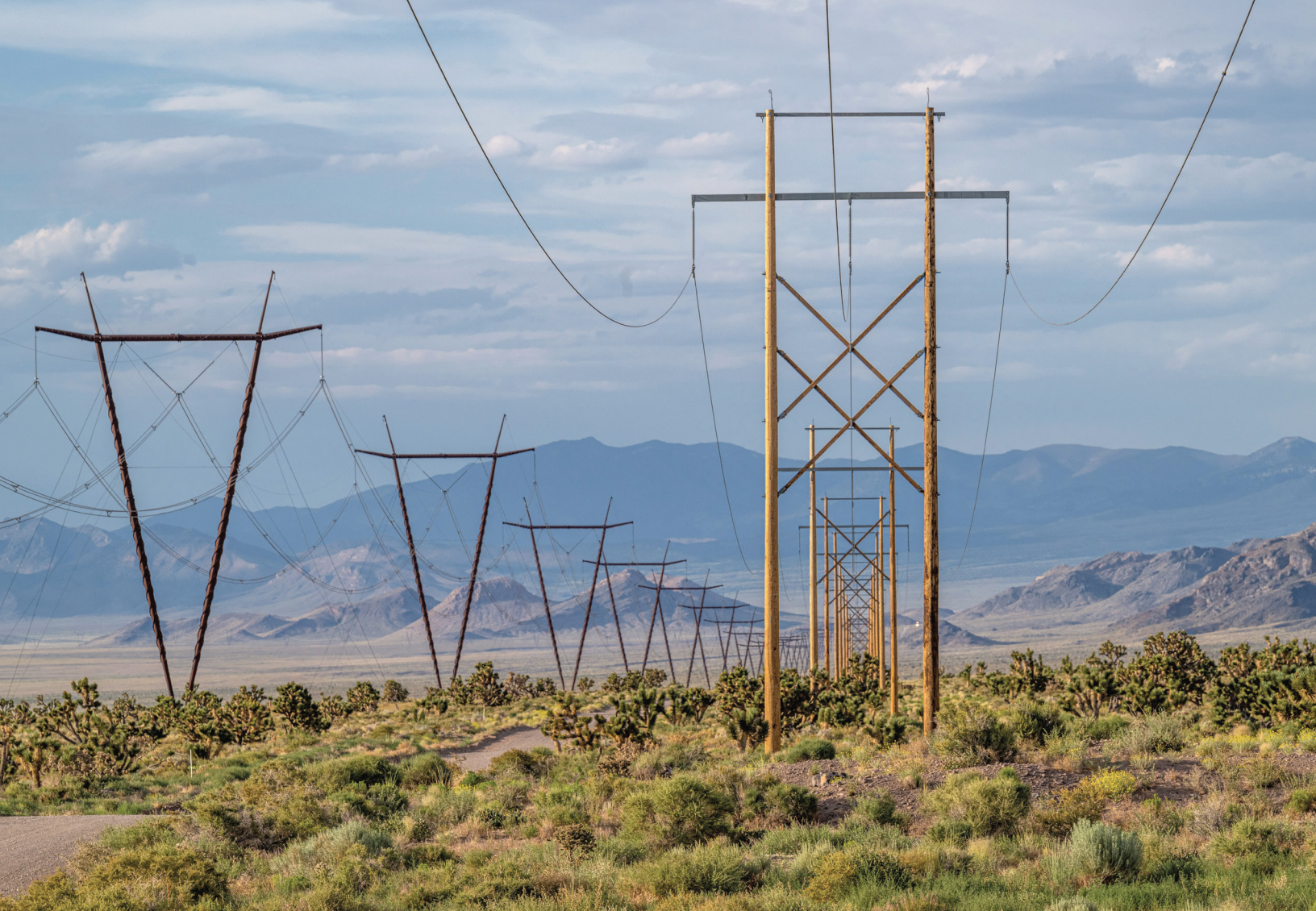
The high voltage One Nevada line and another wooden transmission line run side-by-side in Lincoln County, Nevada. © Bridget Bennett
