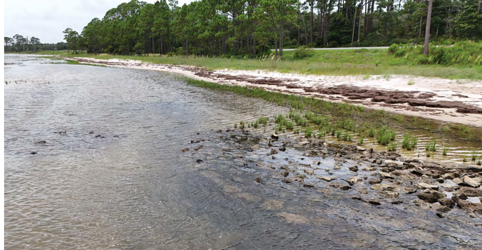
Early installation of saltmarsh plantings and breakwater materials at the Franklin 98 Living Shoreline project (Franklin County). © Darryl Boudreau, NWFWMMD
